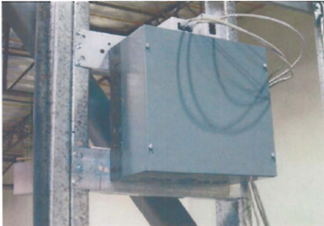
All units were filled with contents and maintained structural integrity and functionality after shake table test
